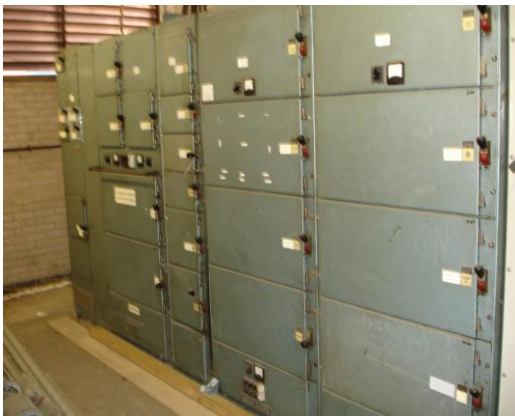
1965 Original LV Switchboard
