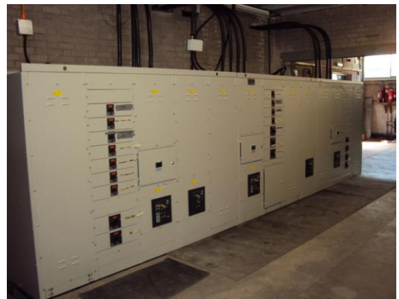
Replacement New Bowers LV Distribution switchboard
