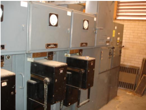
Original Brush VBA oil filled 11kV Switchboard
