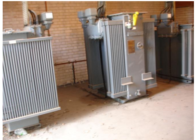
Original 500kVA 1965 Transformers
