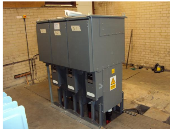
Replacement Schneider Ringmaster SF6 HV Switchboard
