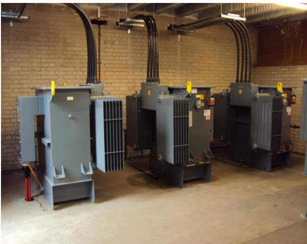
New Bowers 500kVA BEST low loss replacement Transformers installed
